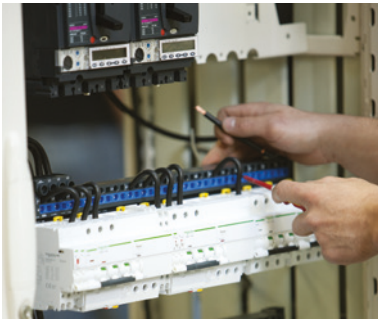
Fig. E30 Assembly of a final distribution switchboard with fixed functional units (Prisma G)
