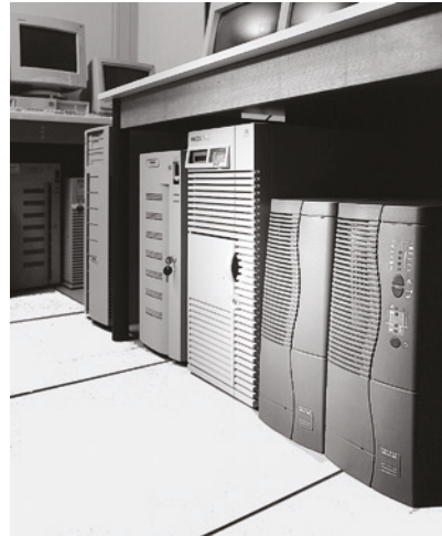
Fig. N32 UPS unit achieving disponibility and quality of computer system power supply
