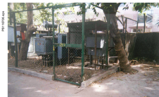
Fig. B53 Outdoor substation without enclosure
